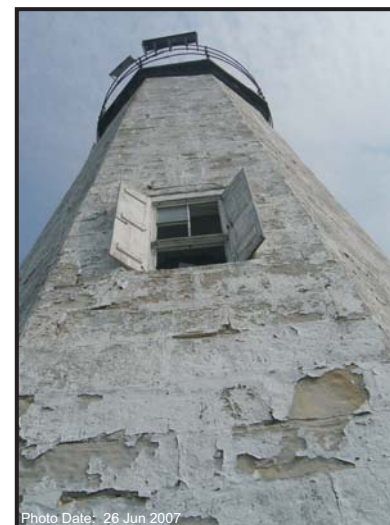
Photo Date: 26 Jun 2007 Peeling paint threatens the integrity of the sandstone structure. The sandstone is being worn away and the mortar between the joints is eroding.
