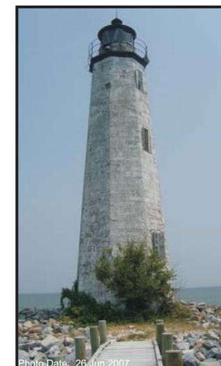
Photo Date: 26 Jun 2007 The small rock size of the present revetment provides little protection during storm events.
